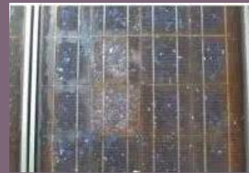
Corrosion of cells in a 15-year-old double-glass module in Hainan (Energy Magazine, 2016)
